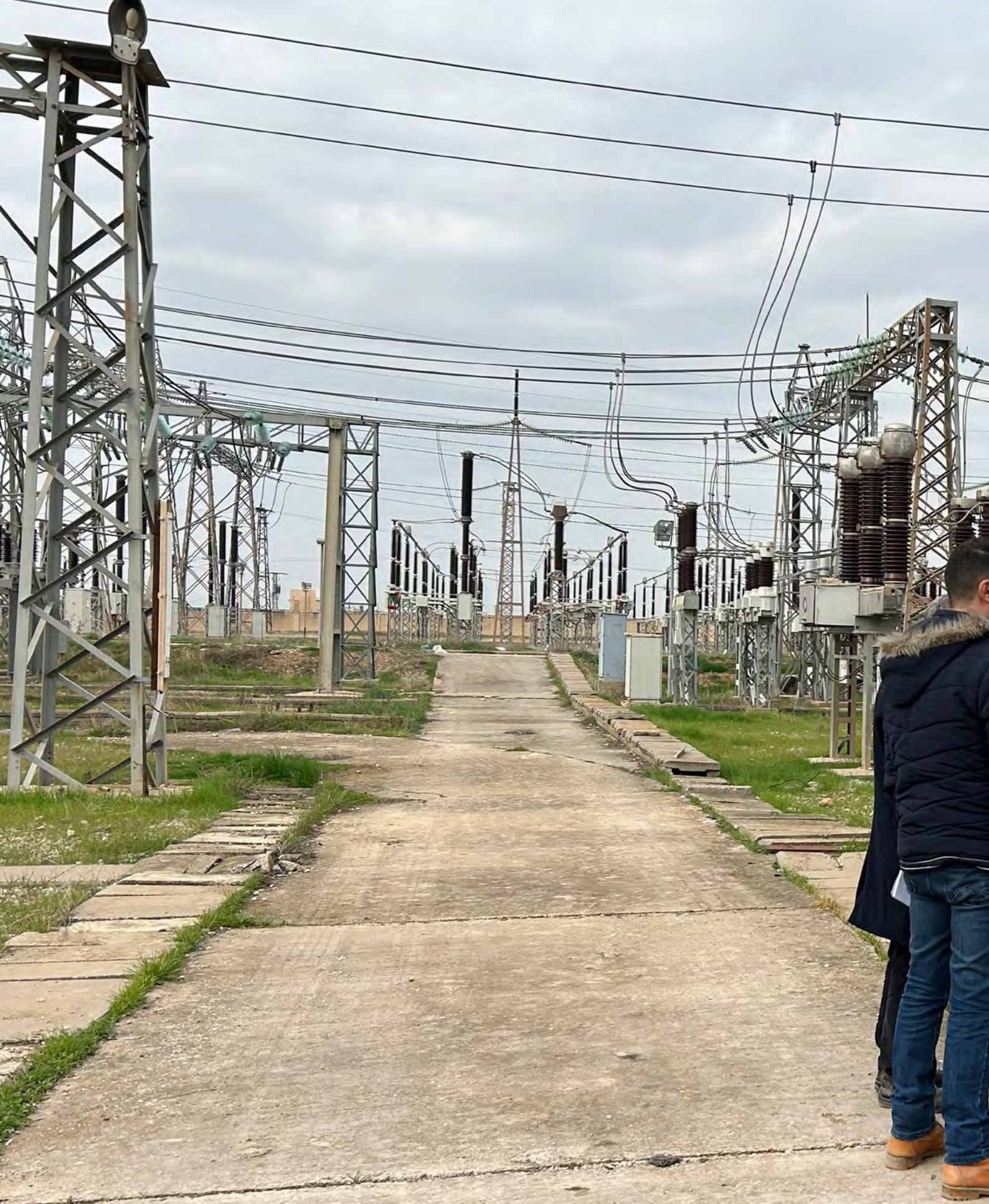
Red Crescent and the public establishment for transporting and distribution of electricity, ICRC staff are carrying out maintenance work at a power station that supplies water pumping stations, health establishments and shops.
